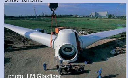
The world's longest blade, the 61.5 meter LM 61.5P is being mounted to a 5MW turbine
